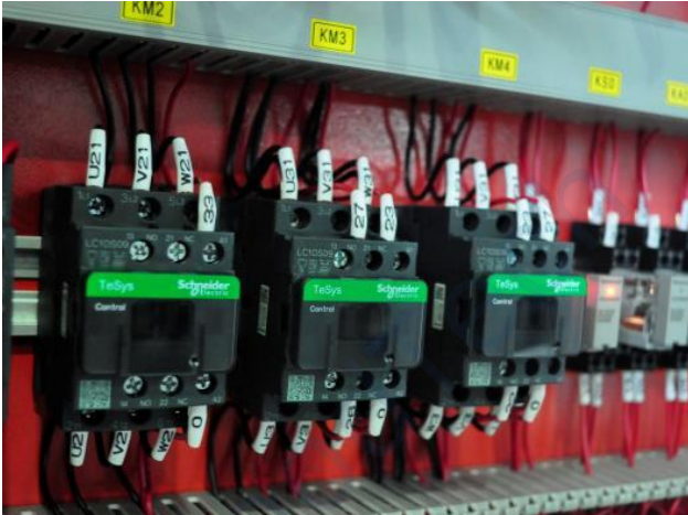
Schneider electrical components and cabinet
